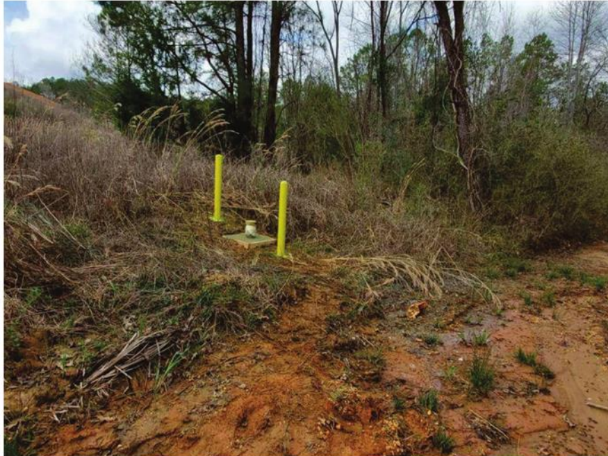
MW-3: Downgradient Well (well protected with bollards and concrete collar – installed February 2023)
