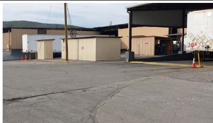
TYPICAL FIXED FOAM SUPPRESSION SYSTEM SHED AT FACILITY (FOAM STATION #2 – SMALL SHED ON THE LEFT)
