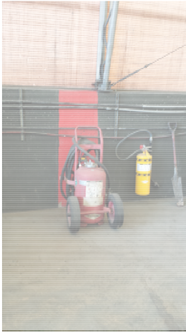
TYPICAL DOLLY MOUNTED CLASS ABC HOSE UNIT AND CLASS D (DRY POWDER) EXTINGUISHER AT FACILITY
